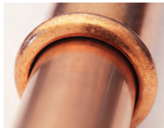
Unpressed fitting - small gap between fitting and tube.
